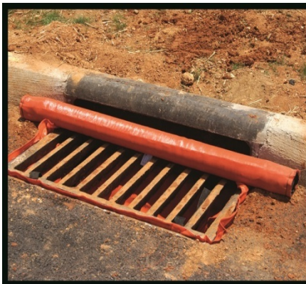
Proper Inlet Protection
