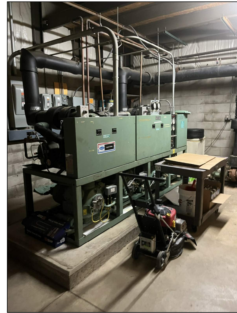
ICE PLANT EQUIPMENT
