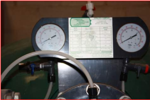
EXISTING DIVING POOL FILTER GAUGES
