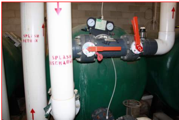
EXISTING SPLASH POOL FILTER (LEFT HAND)
