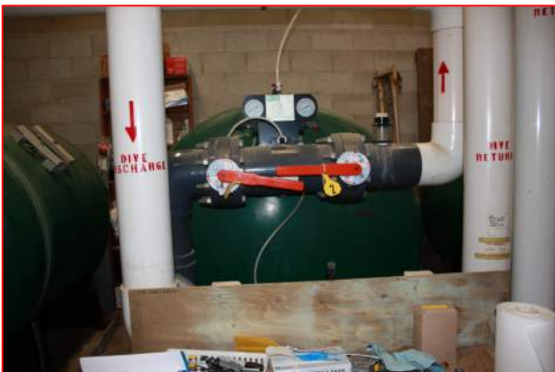
EXISTING DIVING POOL FILTER
