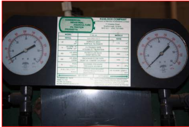
EXISTING SPLASH POOL FILTER GAUGES (RIGHT HAND)
