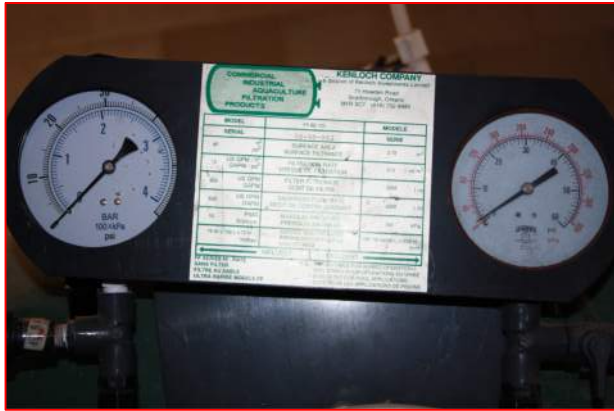
EXISTING SPLASH POOL FILTER GAUGES (LEFT HAND)
