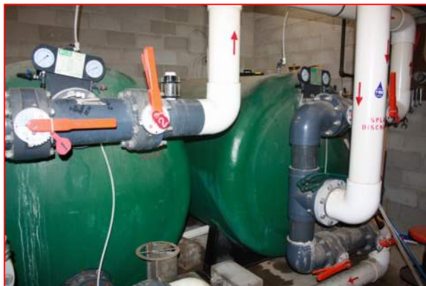
EXISTING SPLASH POOL FILTER (RIGHT HAND)
