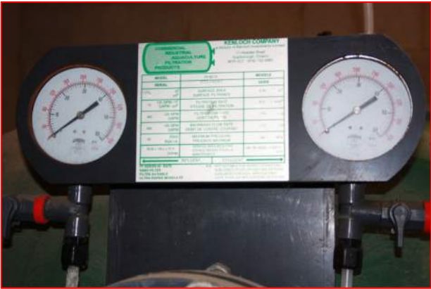
EXISTING LAP POOL FILTER GAUGES
